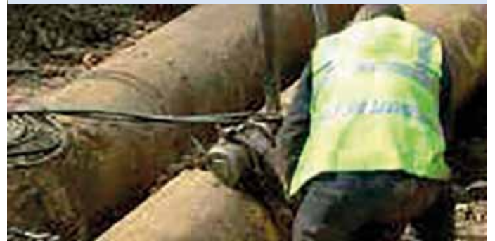
20" Gas main after the Keel Cutters has completed a circumferential cut carried out by a member of the Technical engineers.
