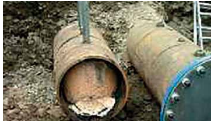
24" gas main following a flow stopping operation and use of the Keel Cutters
